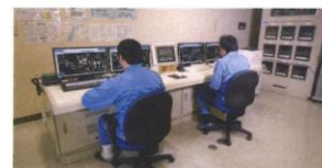
⑩ 中央監視室 Central monitoring room 脱水汚泥搬入から下水汚泥炭化燃料(炭化物)搬出まで施設内の全設備を監視・操作します。 Monitors and operates all the equipment in the facilities, suspending the bringing in of dewatered sludge and discharge of carbonized sewage sludge fuel (carbide).
